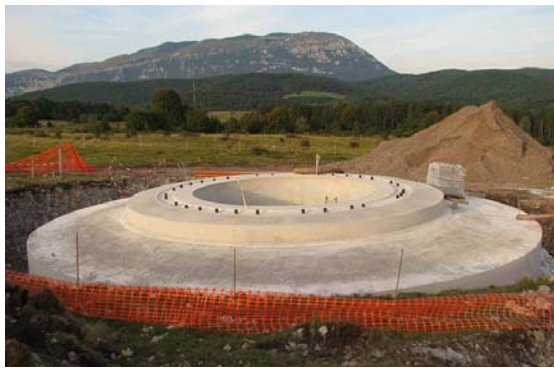
Figure 5. The base of the wind turbine at Dolenja vas [9]
