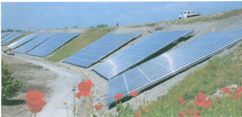
Fig. 2-34: Solar Collectors on a noise protection wall in Crailsheim
